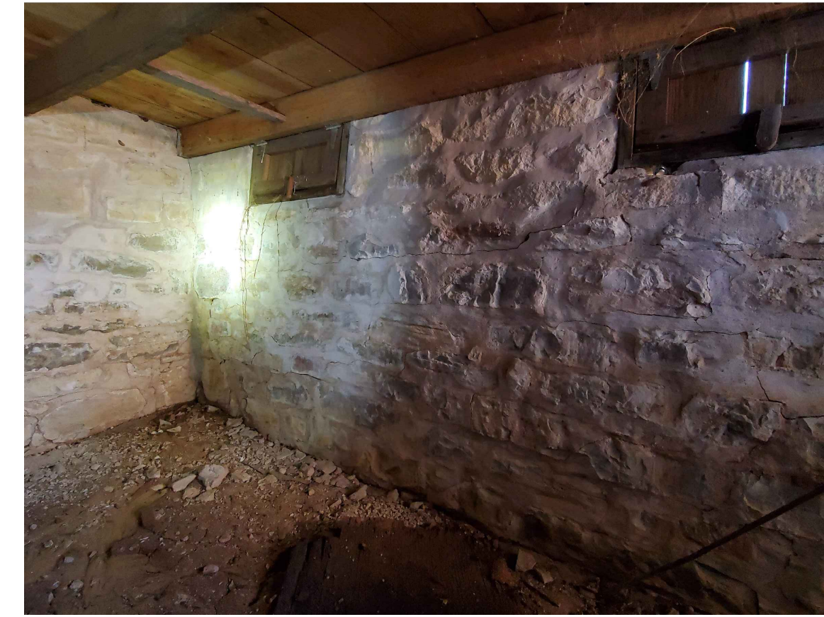
D NORTH CABIN CELLAR SOUTH WALL NO WORK PROPOSED INSIDE CELLAR OTHER THAN TEMP. SHORING IN ACCORANCE WITH KEYED NOTES 2 AND 3 ON DRAWING C-2.
