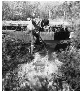
Figure 1. A garden fork is used to dig a trench through the beaver dam.
