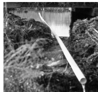
Figure 5. The solid section is in place in the dam; the perforated section extends into the pond in the background.
